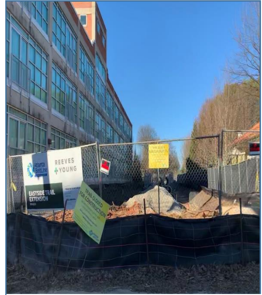
Figure 3: Construction of the Atlanta BeltLine Eastside Trail Southern Extension abutting the Site. Estimated completion February 2019.
